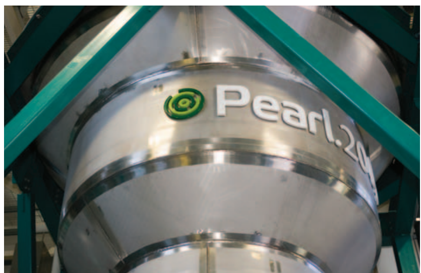
OSTARA TECHNOLOGY IS IN OPERATION AT FIVE WASTEWATER TREATMENT FACILITIES IN THE US. BY THE END OF 2013 THE TECHNOLOGY WILL BE IN USE AT TWO MORE SITES, INCLUDING ONE IN SLOUGH, IN THE UK. THERE ARE CURRENTLY NO INSTALLATIONS IN AUSTRALIA.
